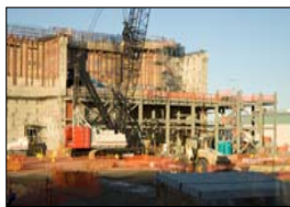
Hanford, Washington Liquid Waste Treatment Plant = US$12 Billion
